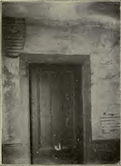
The damp hallway, out of repair
